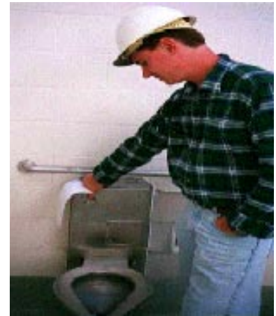
Glenn Leeks flushes one of 500 toilets at the jail, checking for dye.
